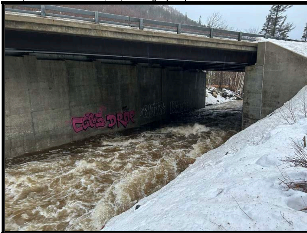
Photo 2: Inlet of NH Route 302 bridge at Saco River Station 24,723 during December 2022 storm event.
